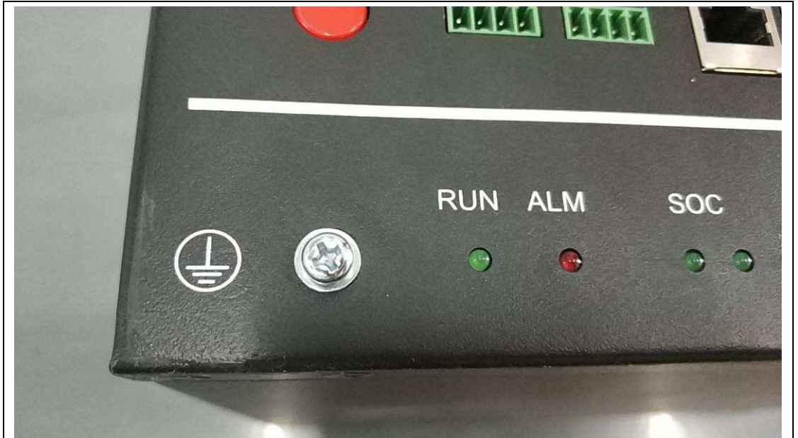
General view of Grounding terminal
