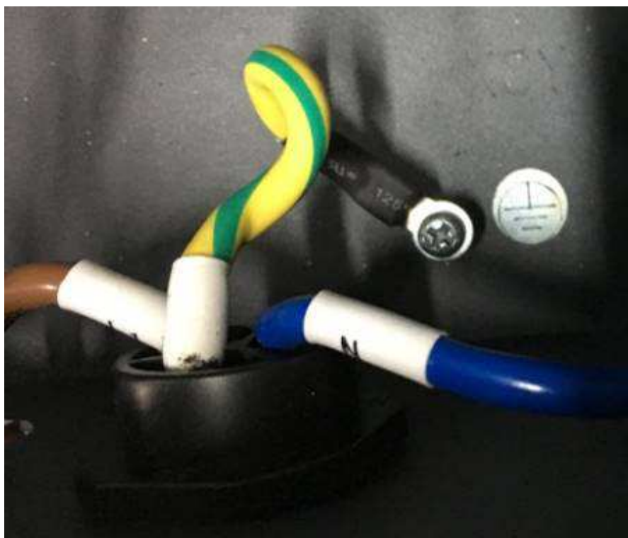
General view of Grouding point
