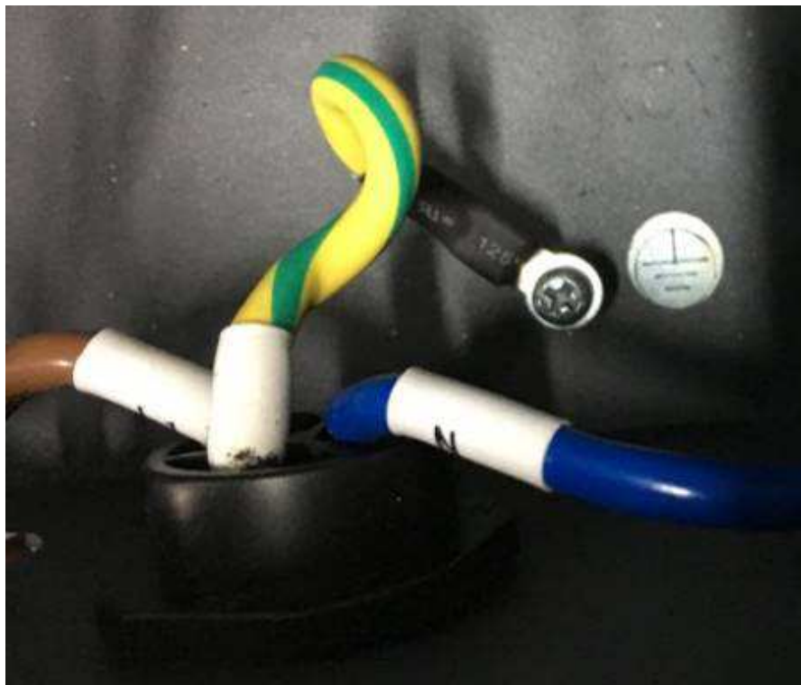
General view of Grouding point
